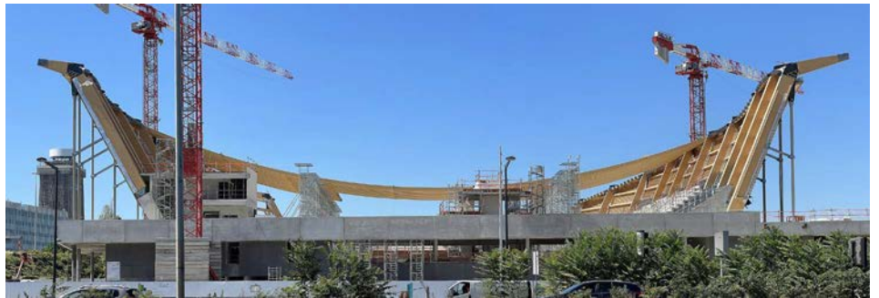
The Paris 2024 Olympic Aquatic Centre is one of the structures discussed. In this construction shot you can see what was at the time the largest wooden hanging roof in the world. Image: CC/Chabe01
