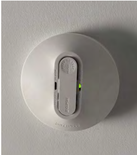
Smoke detectors are an essential part of safety for your home and business. Don't skip on proper care and maintenance. Image: Jessica Hockridge
