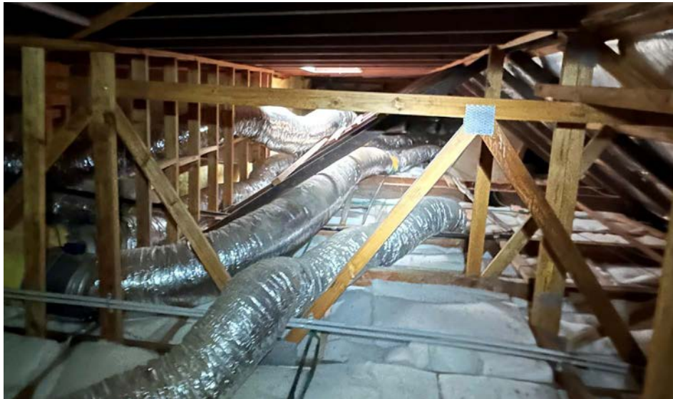
This photo illustrates a classic opportunity for buckling. Photo: Courtesy Paul Davis
