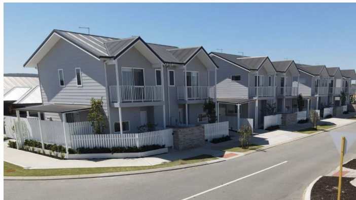
WA's Offsite Construction delivered these seven townhouses to lockup stage in under a month, allowing their client Inspired Homes WA to complete its Sienna Woods development in record time.
