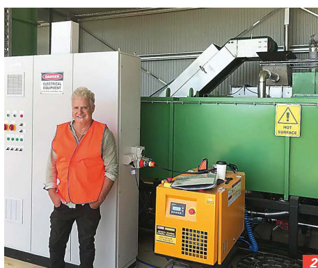
1/ Ricky Dent from Earth Systems jumped at the chance to install biochar technology so near to home.
