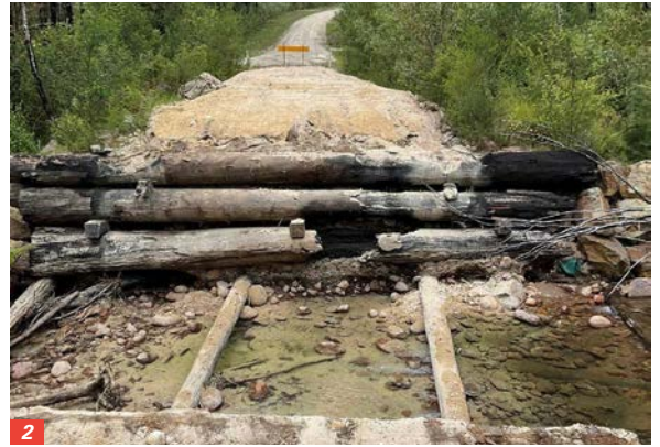
2/ Mountain Road was in need of a replacement bridge and the works have now commenced.
