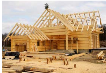
The increased take up of timber will be important to solve Australia's housing crisis.
