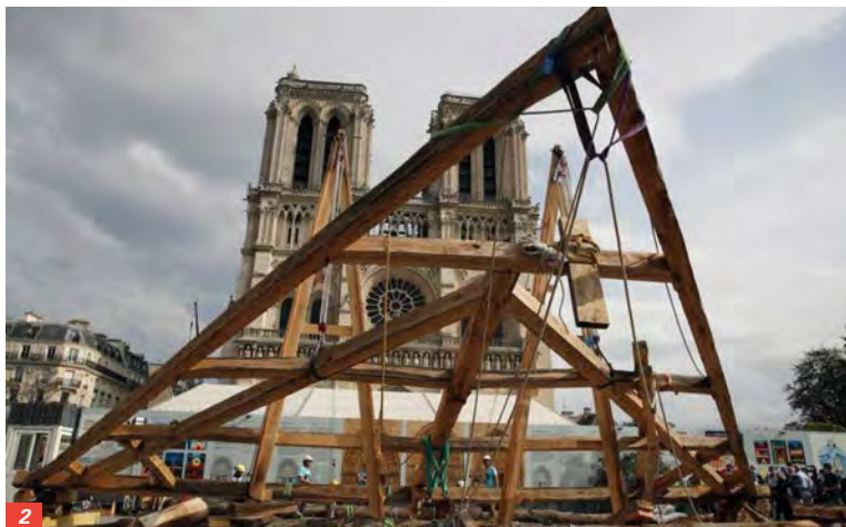
1/ Medieval techniques have been used by carpenters working on the roof restoration.
