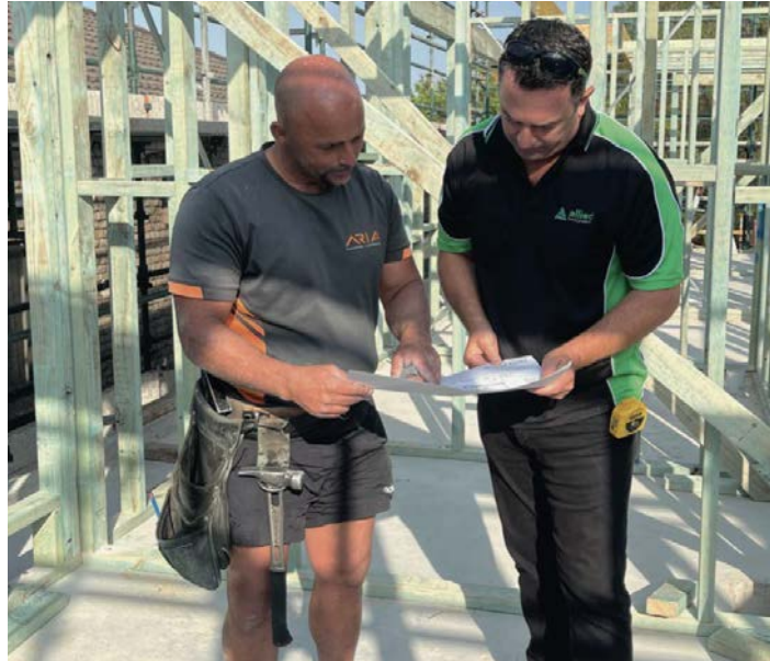
L-R: Milan Timotic, of Aria Carpentry with Adam Krkac providing customer support on site. The new allSYSTEM floor systems are providing assurance and convenience for multi-storey builds.
