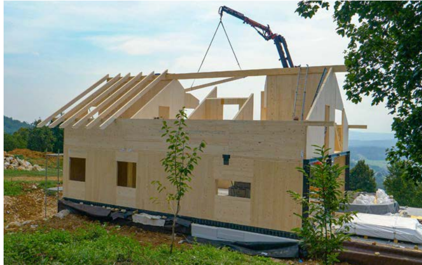
Prefabricated homes go up quickly on site with minimal interruption to the neighbourhood and can usually have their substructures adapted to suit the site. Image: Shutterstock
