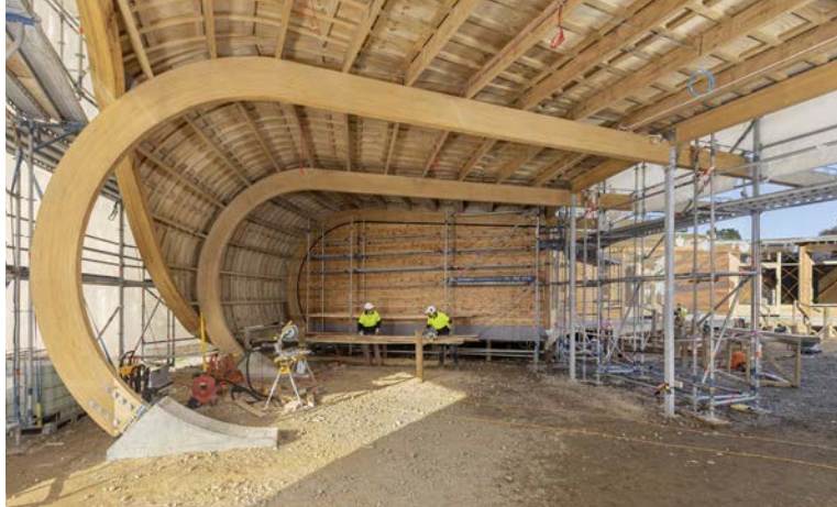
Green School shell under construction. Main contractor: Livingstone Building. Photo: Tania Niwa
