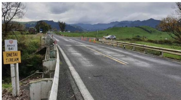
Onetai Bridge is about halfway between Paeroa and Kopu on State Highway 26. Image: Waka Kotahi via NZ Herald
