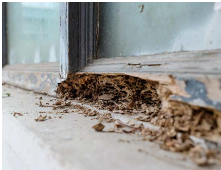
Termites can attack and destroy any unprotected timber parts of a home, even bypassing protected timbers lower in the building, such as on this window frame. Photo: Shutterstock/Atterpon Thana
