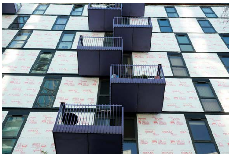
Unsafe cladding is being removed, but too slowly in NSW. Photo: Shutterstock/Fred Duval
